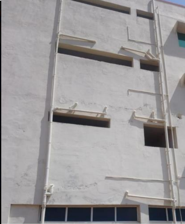
Figure 9 Waster water Pipe from A block
