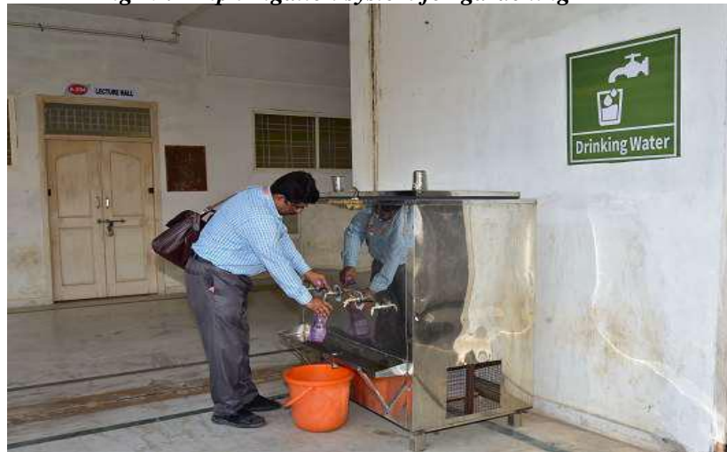
Fig 20: Drinking water connection directly from RO plant (distribution)
