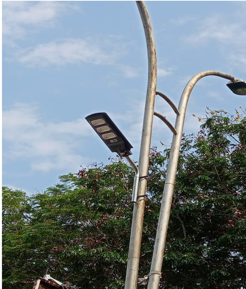
Fig: Solar Panel with Sensor lights at entrance
