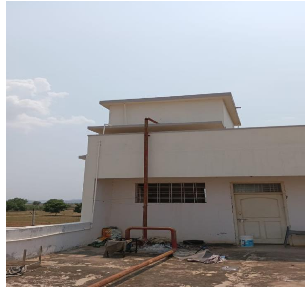
Fig 12: overhead water tank at Canteen
