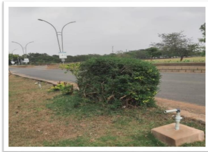
Fig 16: Water distribution utility System in campus
