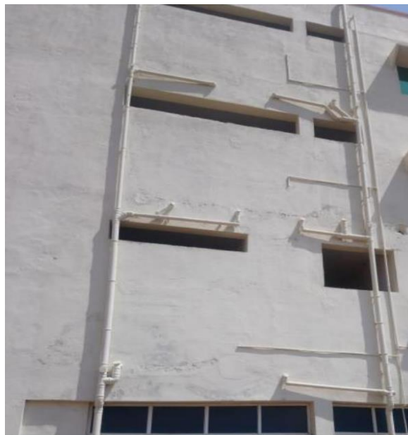
Figure: Waste water Pipeline
