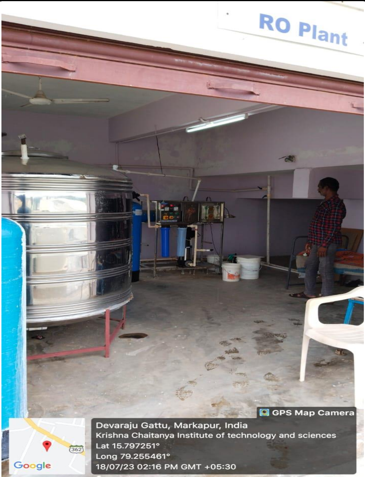
Fig 21: RO plant in KITS campus
