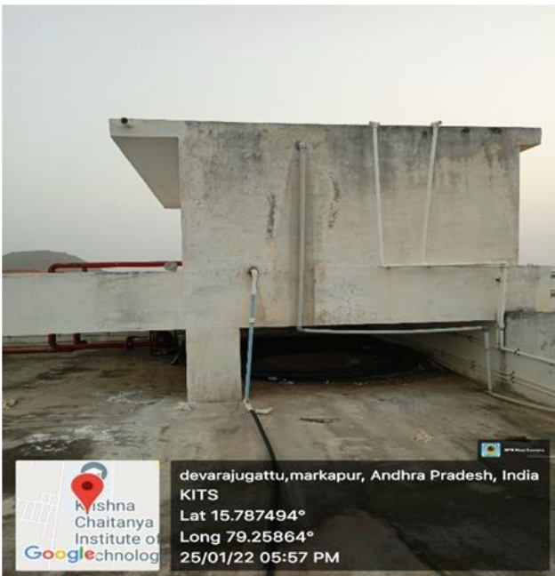
Fig 13: overhead water tank at Block C
