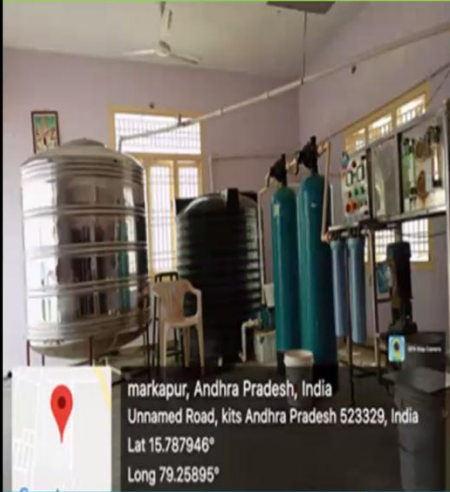
RO water plant providing drinking water
