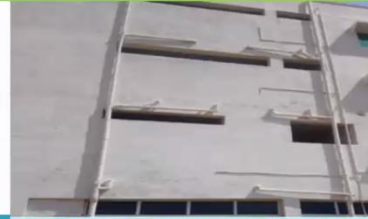
Rain and Waste water outlet pipes, A-Black
